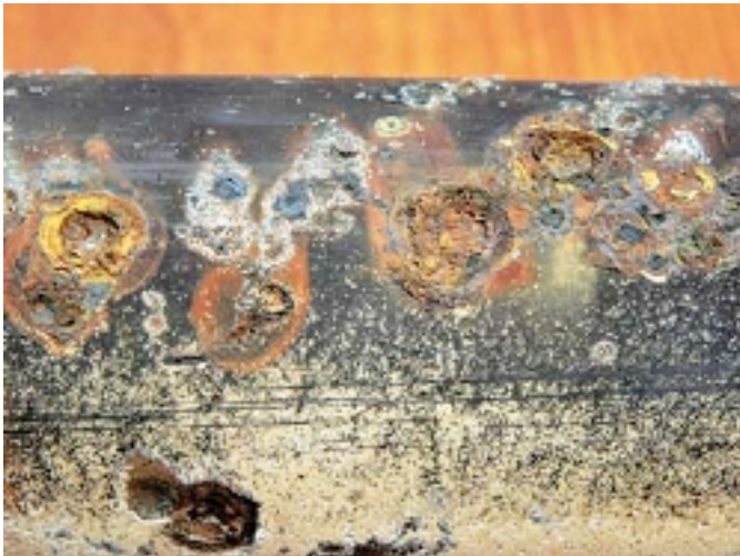
Oxygen pitting on a boiler tube.
