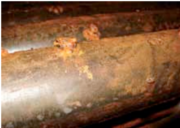
Oxygen corrosion covered by tubercle.
